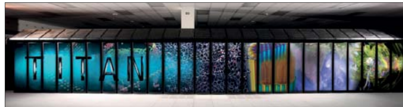
↑ The Cray Titan, currently the world's most powerful computer, has a massively parallel architecture built from surprisingly mainstream CPU and GPUs
